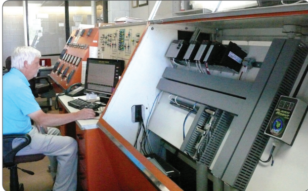
Jim Laford, division supervisor of Amherst's Wastewater Division, works in the main water treatment plant with the safety and security of AlarmAgent.com
